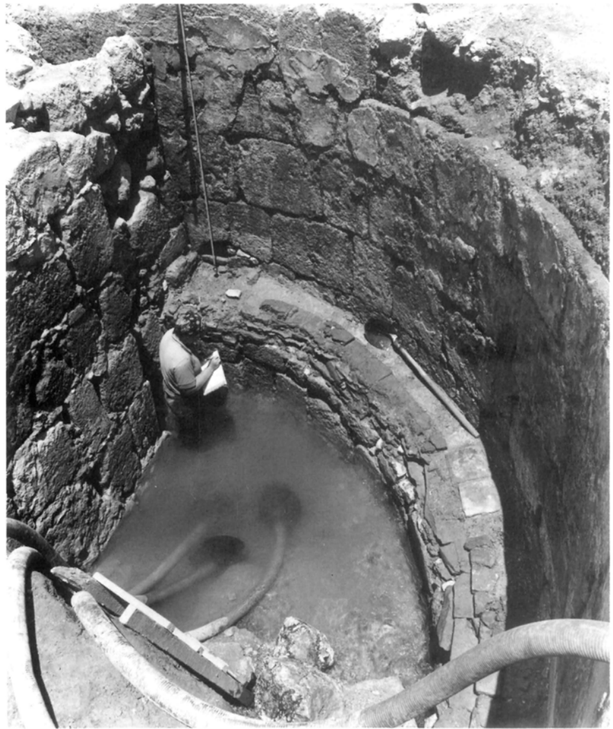
Figure 4: Excavations of the bath building, showing pipes pumping out the water while excavation is carried out. Photograph: Pella in Jordan 2, Plate 85.
