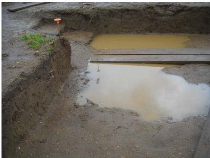
Torrential downpours on the site: digging still continued. Image: Helena van der Riet.
